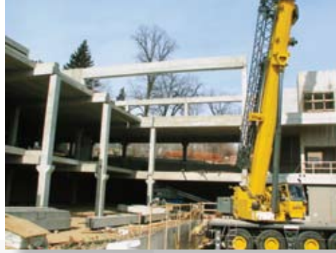
A precast concrete structural frame provides the building's complete skeleton. Photo: Molin Concrete Products Co.
